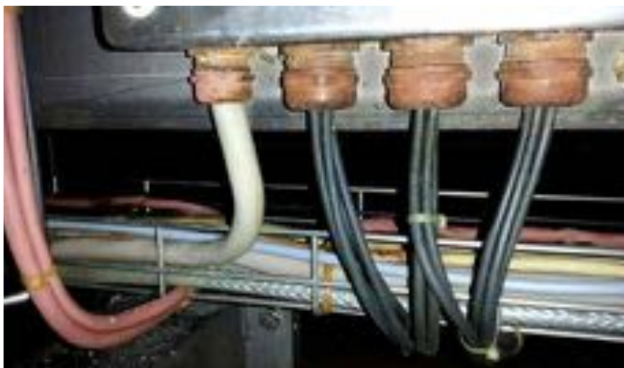
In the food and beverage industry, cables and cabling components are subjected to particularly strenuous conditions. If unsuitable components are used, then screw joints could corrode and the cable insulation could swell, as can be seen in the image. The components would lose some of their functionality and it could result in hazardous situations.
